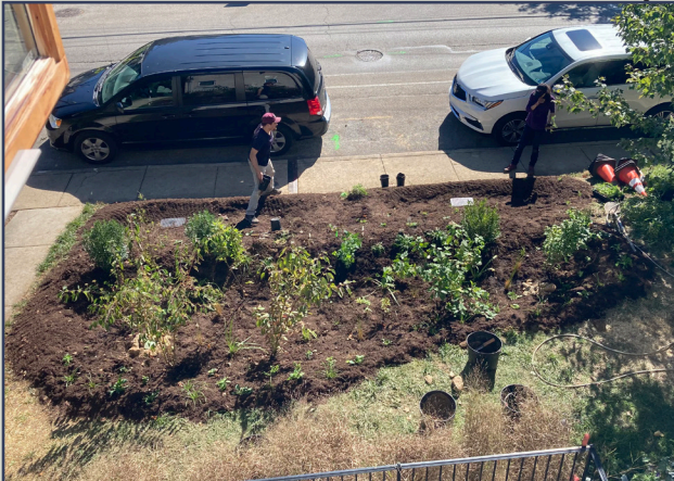
An overhead view of a new Narberth rain garden.
