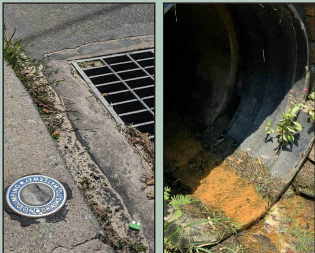
Left: Signage alerts people that the sewer drains directly to waterways. Right: Iron bacteria on the bottom of a stormwater outfall.
