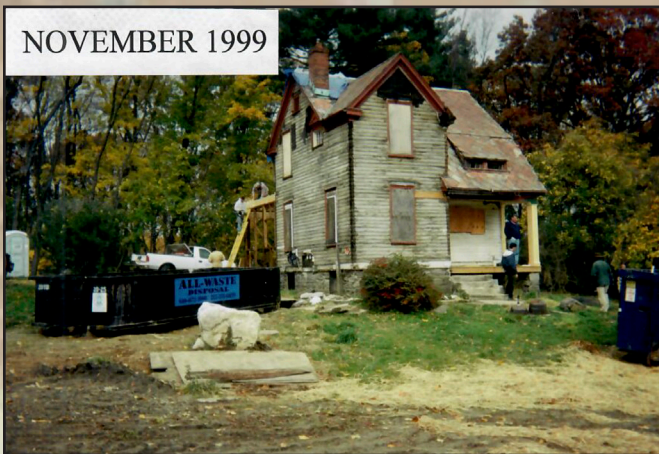
In 1998, LMC commissioned the architectural firm of Atkin, Olshin, Lawson-Bell and Associates.
