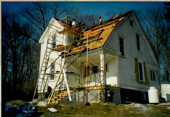
A feasibility study of the Cottage's structural soundness and its ability to meet our office needs was conducted.
