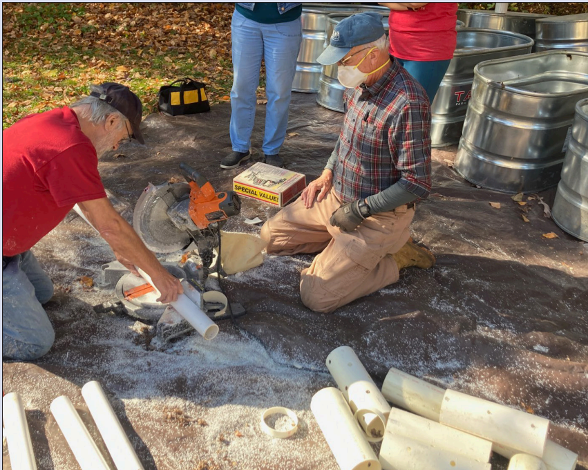
Cobbs Partners come together at the Conservancy Cottage to assemble downspout planters.
